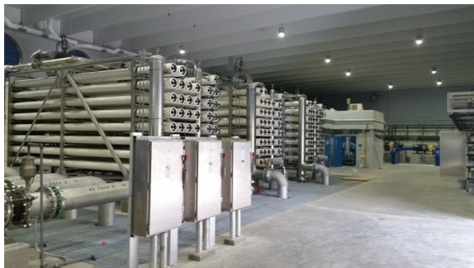
A brackish groundwater treatment facility constructed in Clearwater with cooperative funding by the District
