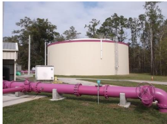
Reclaimed water storage tank in Brooksville
