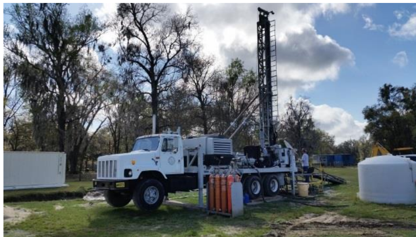
The District's ROMP program exploring the Lower Floridan aquifer in Sumter County
