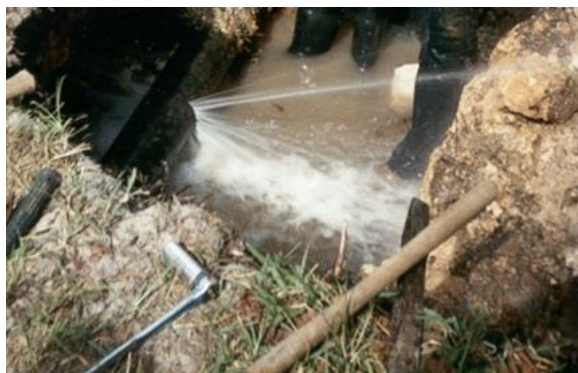
The District performs leak detection surveys in an effort to reduce water loss.
