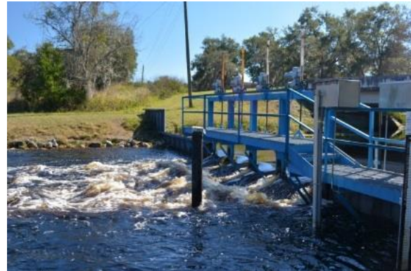
Control structure at Tsala-Apopka Outfall
