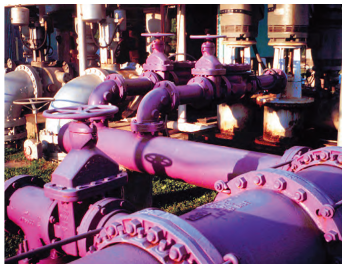
A reclaimed water pump station.
