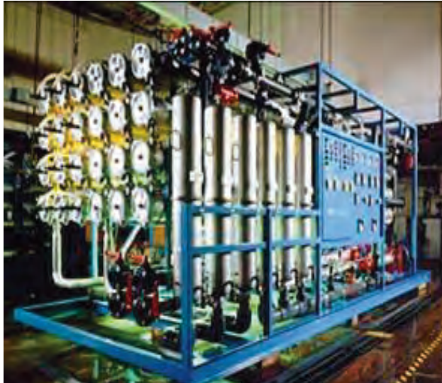
A reverse osmosis system for desalination of brackish groundwater.
