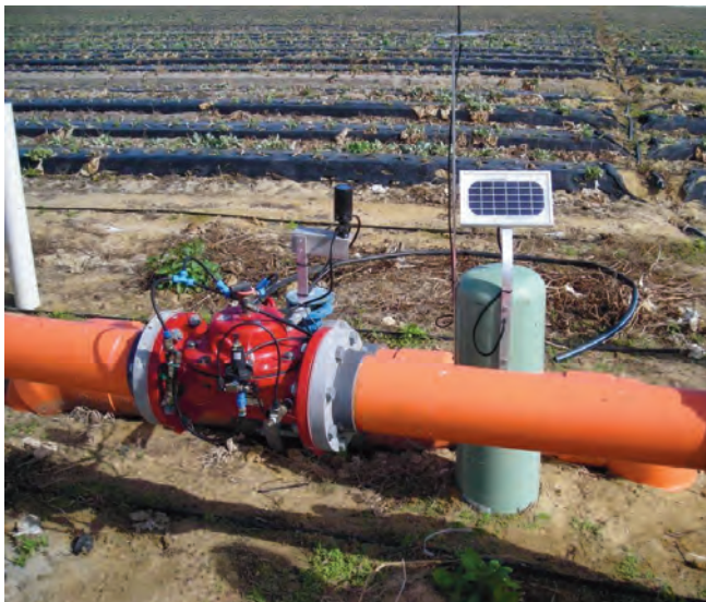
The FARMS Program provides funding for growers to install water-saving technologies such as this solar powered, remotely operated valve on an irrigation system. The District classifies FARMS as water resource development.
