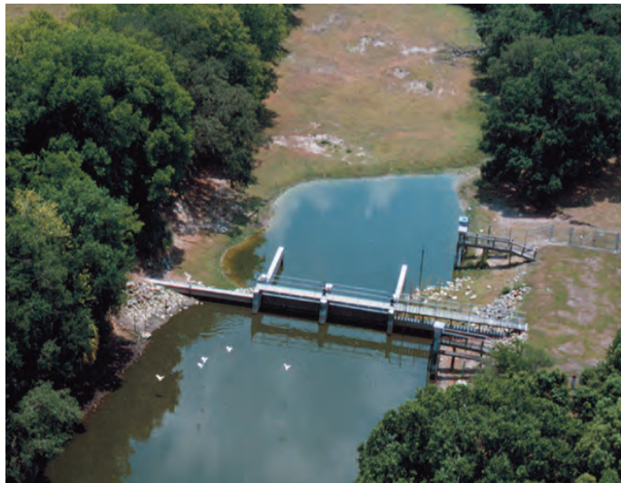
The Lake Hancock Outfall Structure (P-11) will be rebuilt to enable water levels in Lake Hancock to be maintained at higher levels.
