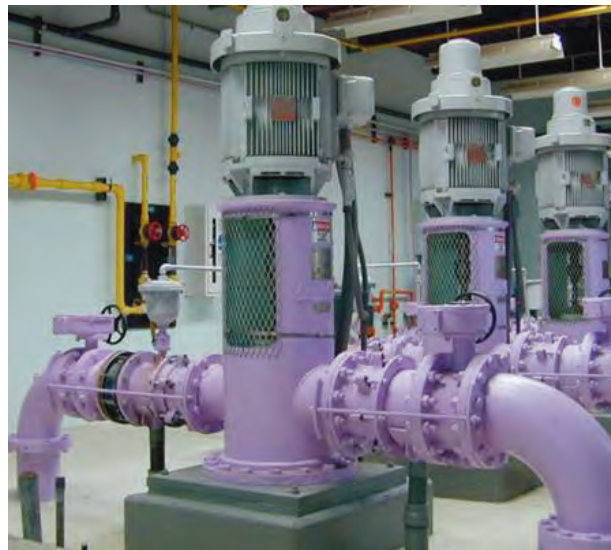
A reclaimed water pump station.
