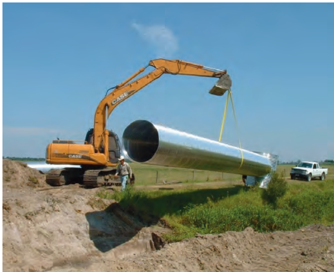
Installation of a water control structure as part of a tail-water system that will capture and reuse agricultural irrigation water.
