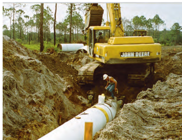
Construction of a potable water transmission pipeline funded in part by District matching funds.
