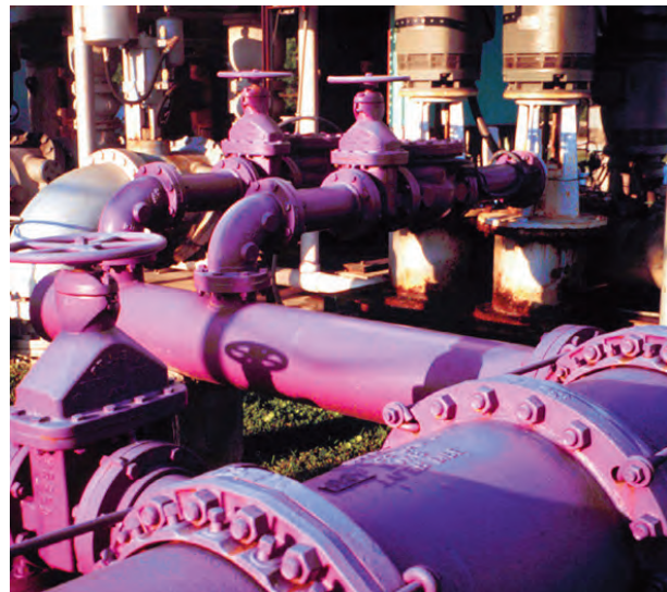
A reclaimed water pump station.
