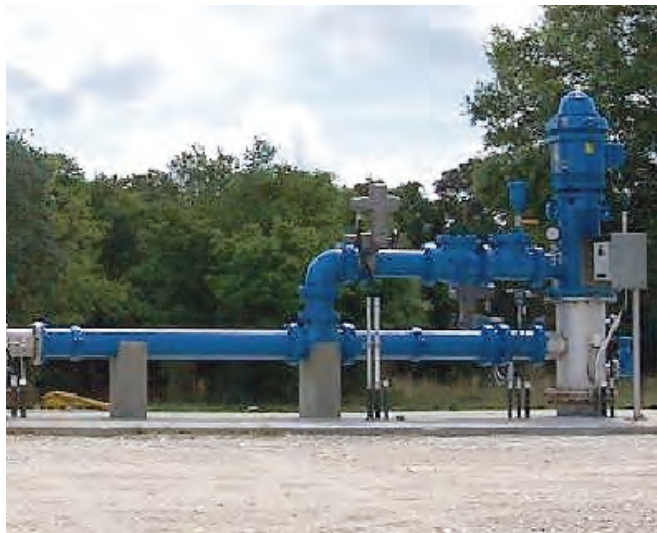
One of the Peace River Manasota Regional Water Supply Authority's operational aquifer storage and recovery wells at the Peace River facility.
