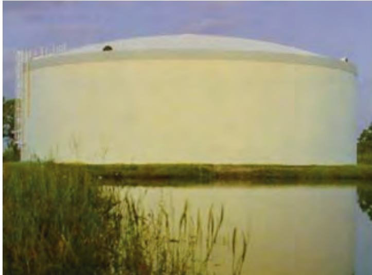
Reclaimed water storage tank.
