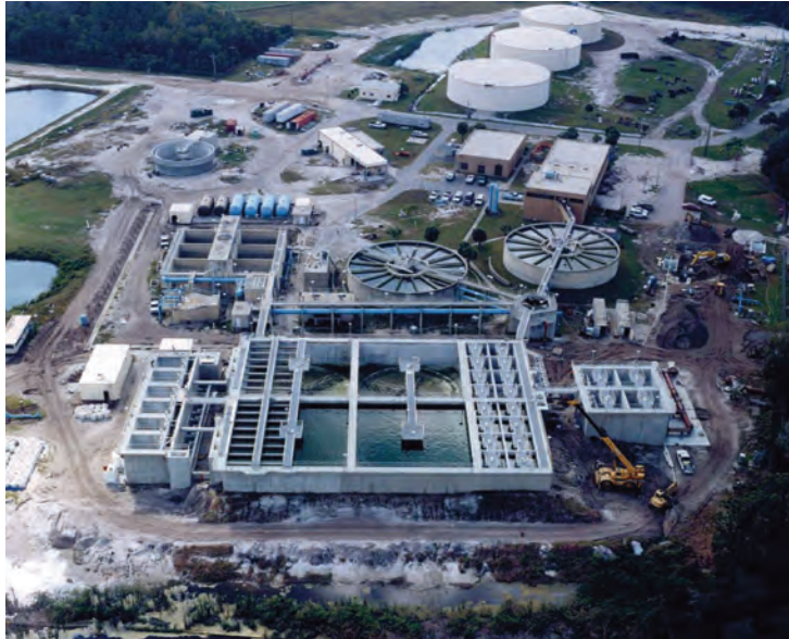
Construction of an early phase of the Peace River Manasota Regional Water Supply Authority’s water treatment plant at the Peace River facility in DeSoto County.
