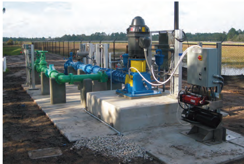
An aquifer storage and recovery well.
