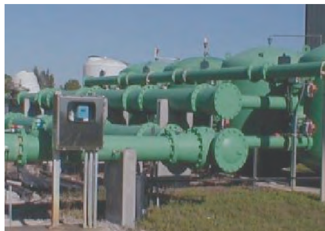
The pre-filtration system of a brackish groundwater desalination facility.
