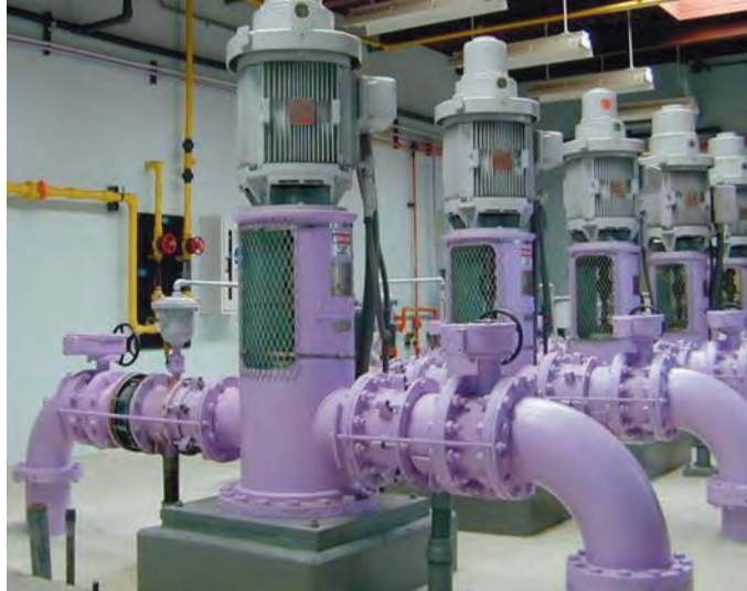
The District has provided hundreds of millions of dollars in matching funds to local governments to develop water supply infrastructure such as this reclaimed water pump station.
