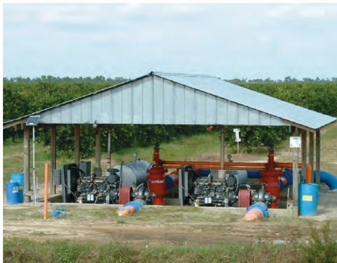
The District partners with state and federal agencies to provide cost-share funding and technical assistance to growers to install water-saving technology such as this tail-water recovery system for a citrus grove.
