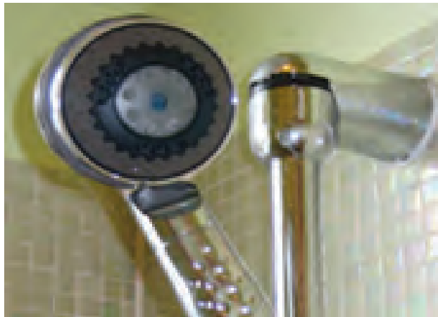
The District assists utilities with the development of incentive programs that encourage their customers to install water-saving fixtures such as low-flow showerheads.
