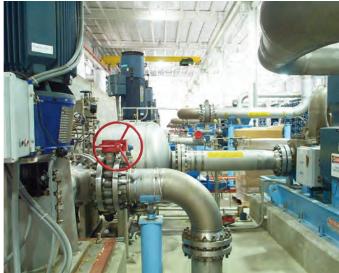
An interior view of the Tampa Bay Seawater Desalination Facility.
