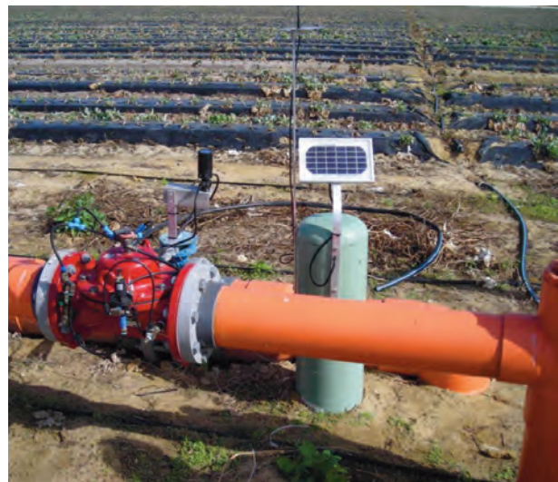
The FARMS program provides funding for growers to install water saving technologies such as this solar powered, remotely operated valve on an irrigation system. The District classifies FARMS as water resource development.
