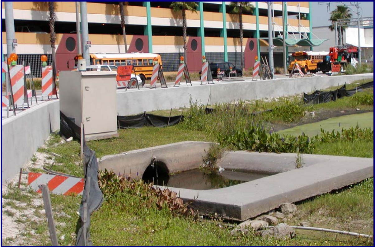
Picture 2 – Inflow and sedimentations basin during trolley construction and pond reconfiguration. Finished parking garage is in background.
