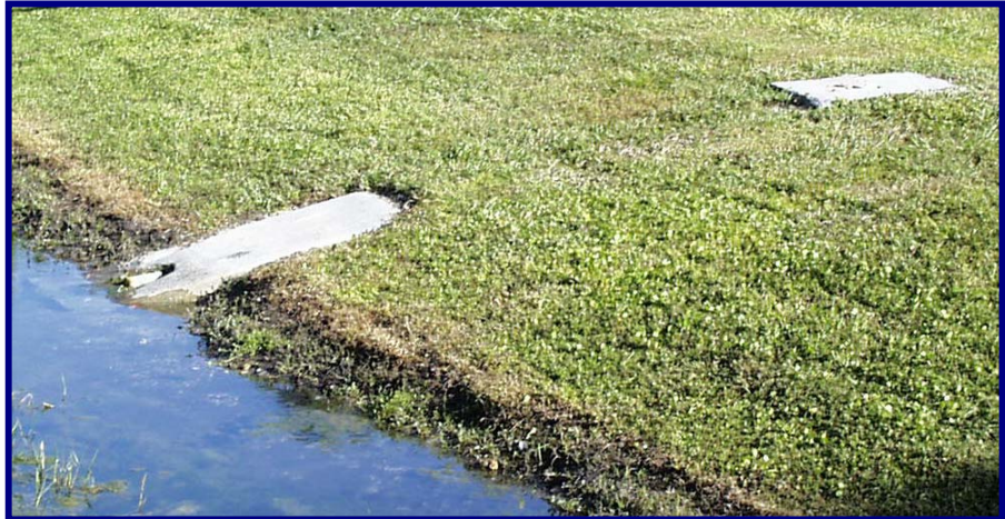
Picture 4 – Underdrain intake and cleanout.
