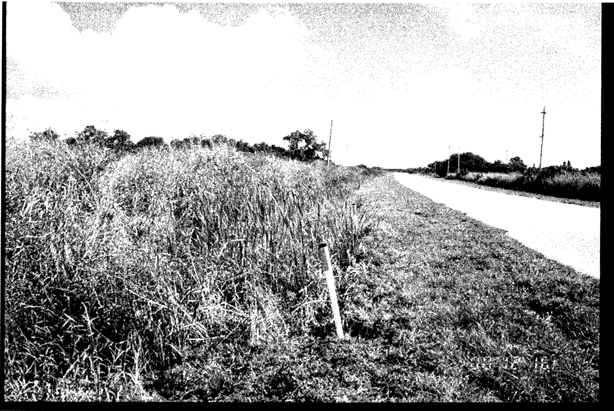
Ditch at station (site 2 SED1). Right before runoff flows under the road and into the pond. Shows the overgrown vegetation in the ditch.
